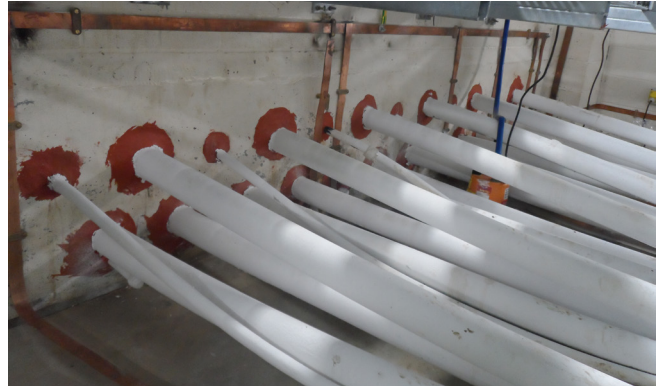
Leaking mastic sealing solution
