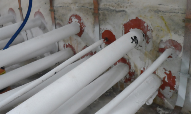
Leaking mastic sealing solution
