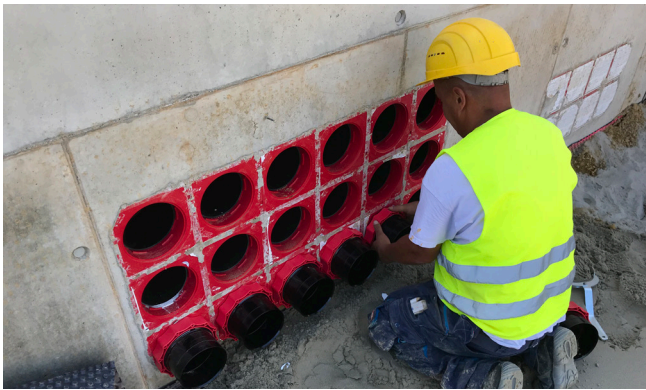
Installation of system cover HSI 150 – M168 WR in preparation for later connecting the corrugated cable duct
