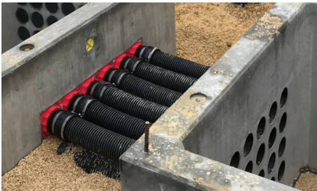
The connection between shafts was made by using factory-installed ducts, HSI 150 wall inserts and our HSI 150 – M168 WR system cover.
