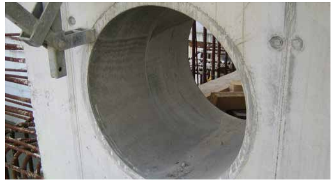
FZR400/300 – installation in water treatment plant
