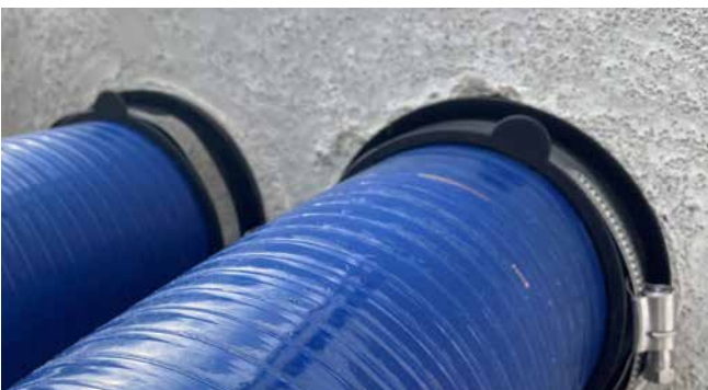
HSI150 KMA installed
